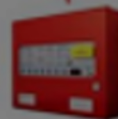
Fire Alarm Control panel
